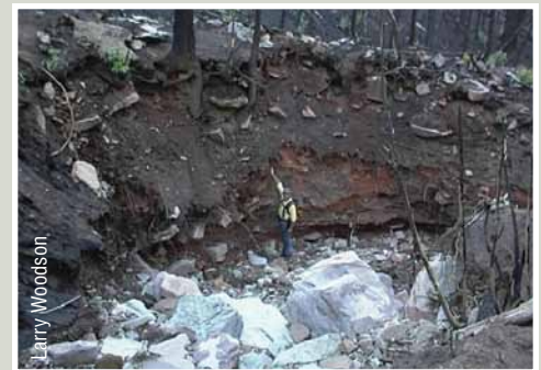
Serious erosion after the Missionary Ridge fire damaged water quality, flow regimes and aquatic habitat.
