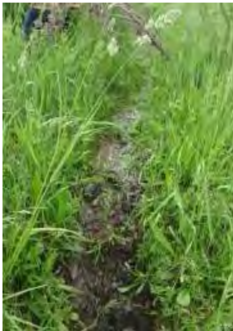
Photo 21: Water overtopping levee from Wetland B into Wetland A, 5-29-13.
